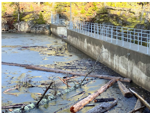
Arrowsmith Dam – Debris accumulation
